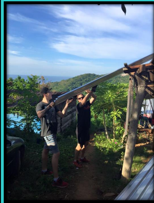
Tony and Tyler helping with the sheeting, watch out for those scorpions
